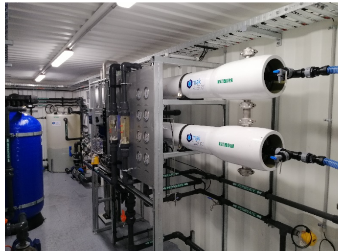
MAK Water containerised SWRO plant installed onsite
