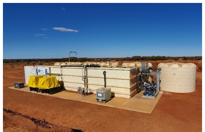
Internal view of the containerised SWRO plant
