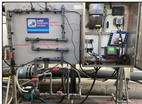
WTS 5-0017 onsite dosing skid with monitoring equipment
