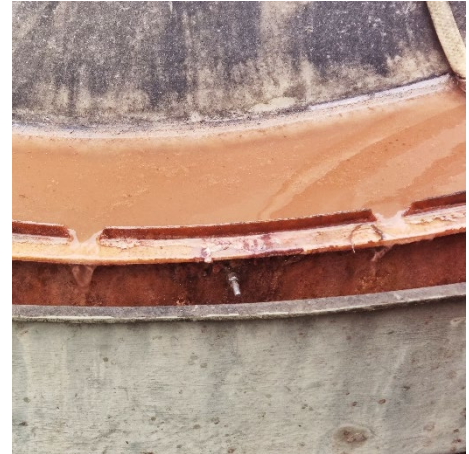
Turbid DAF effluent before application of WTS chemistry solutions
