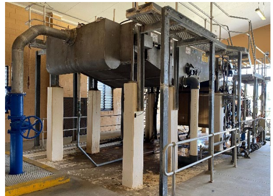
Belt Filter Presses at one of the sites
