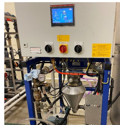
Polymer preparation and dosing system installed at one of the site to make up and dose the polymer + flocculant solution
