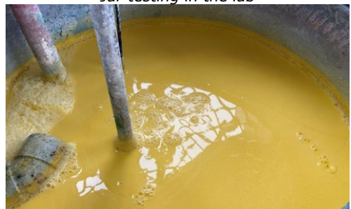
Onsite mixing and dosing tank
